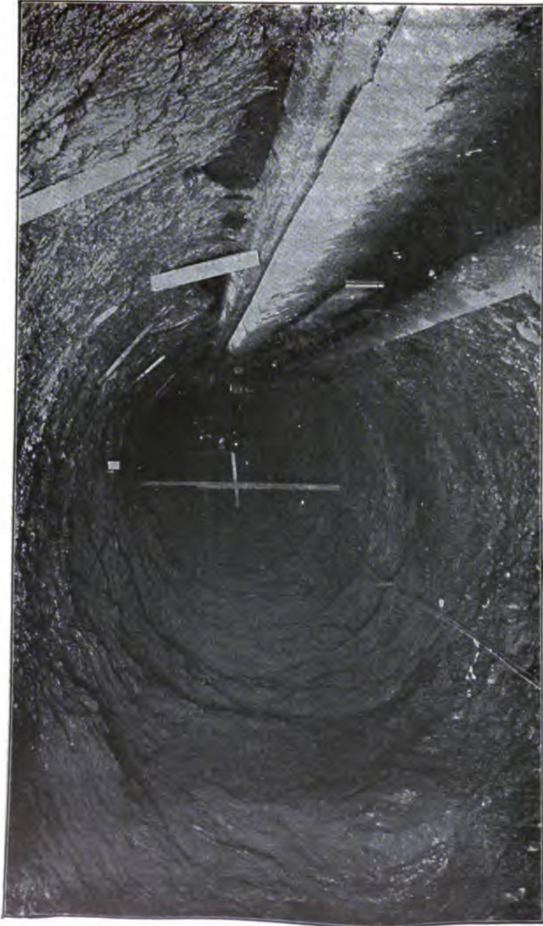
PLATE 100.—Contract 12. Trimmed Tunnel in Hudson River Shale and 5-foot Strip of Invert as Laid for Rondout Siphon. This invert affords a foundation for tracks and forms.
